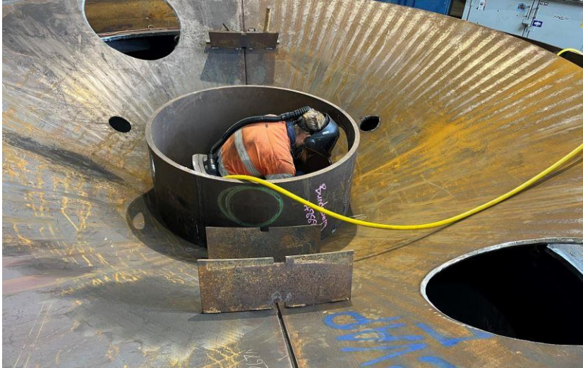
A Wilmar boilermaker fabricates the bottom cone for one the evaporators being manufactured at the Burdekin Centralised Workshop.
