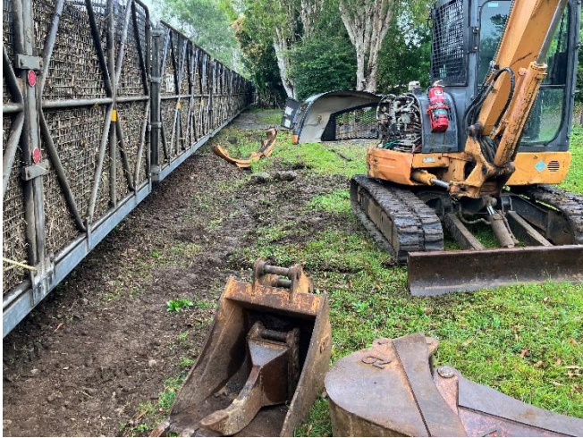
An excavator sustained significant damage when it collided with a cane train at Proserpine.
