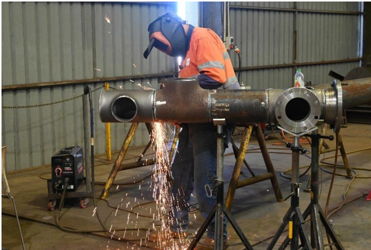
CAPTION: A Wilmar boilermaker constructs the juice pipework associated with the Victoria Mill evaporator project.
