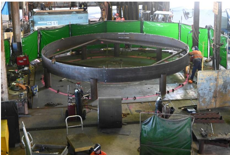
CAPTION: Fabrication of the bottom cone section of the new evaporator for Wilmar's Victoria Mill.
