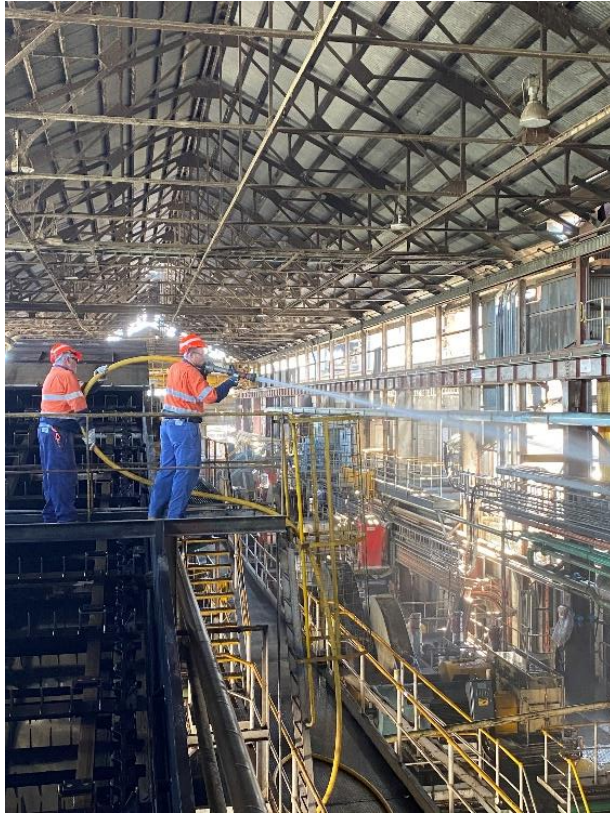
CAPTION: Terry Brown (left) and Justin Benato wash down the milling train at Wilmar's Pioneer Mill.
