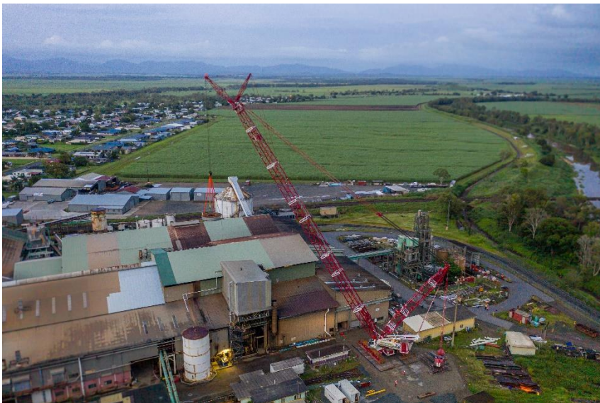
A 600-tonne crane with a superlift on the back was used to lift the pan components through the roof of Proserpine Mill.
